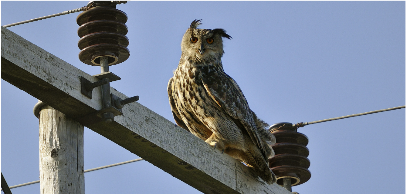
Eagle owls are frequently resting at the power line pole cross arms, exposing themselves for electrocution hazard. Photo: Frode Johansen
