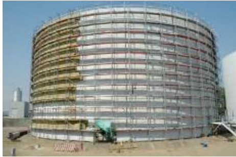
District heating, Theiß, Austria
