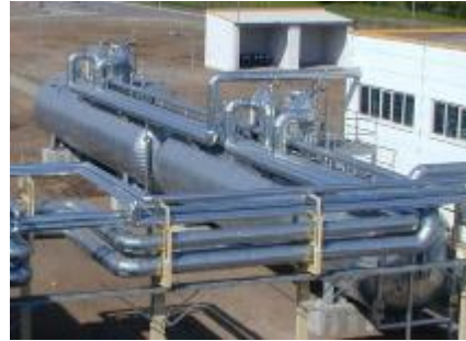
Steam accumulator, Aerated concrete manufacturing
