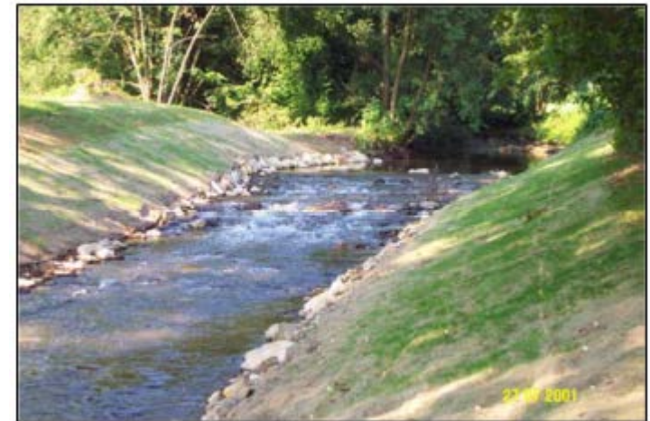
Figure 8. Rockfilled slide in the Aich River (LUBW, 2005)
