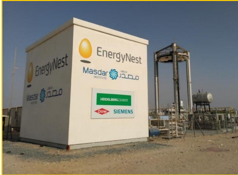
EnergyNest TES pilot installation in Masdar City, Abu Dhabi, UAE.
