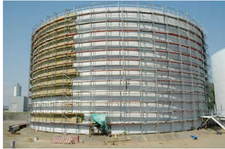
District heating, Theiß, Austria
