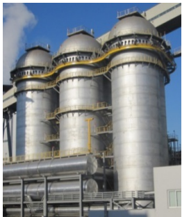
Cowper storage, blast furnace industry >500\text{ }^{\circ}\text{C}
