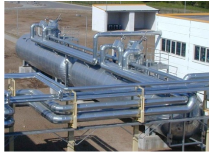
Steam accumulator, Aerated concrete manufacturing
